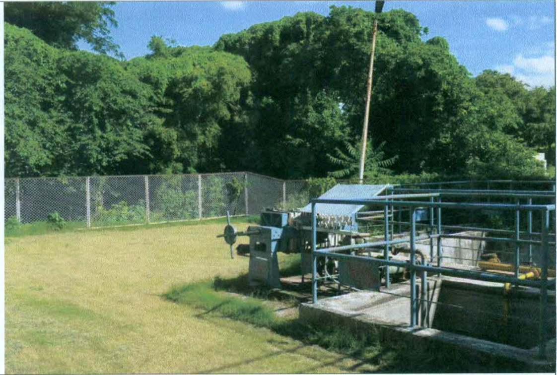
SEWAGE TREATMENT PLANT
